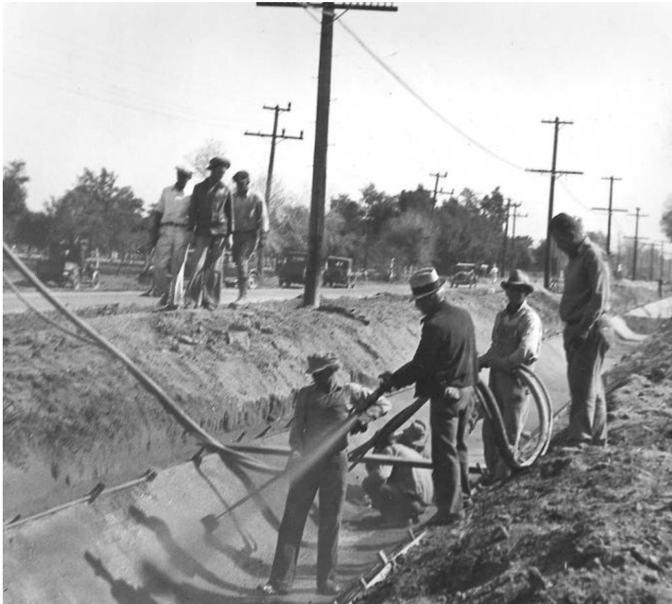
Chapter 7 - Figure 19: Photograph of Civil Works Administration workers applying cement with a power gun on a construction project in Phoenix, 1934. Arizona State Library, Archives and Public Records. History and Archives Division, 98-3571 .
