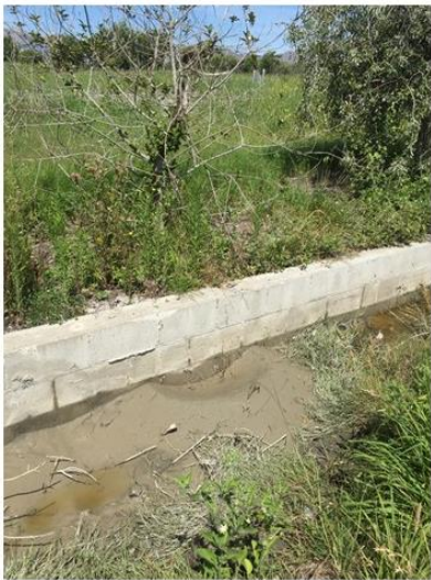
Figure 6. Wall separating Bexley South and Bexley Central. A liquefaction feature is observed on the Bexley Central side of the wall that has a thinner non-liquefiable crust.
