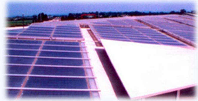
PHOTOVOLTAIC PANEL ON ROOF
