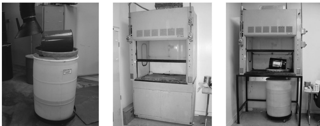
Figure 2. Original flexible exhaust line (left), original fume hood configuration (center), and retrofitted fume hood—note modification to easily roll drum underneath for safe bulking (right).
