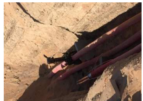
Figure 2.3.7 more than one cable in trench
