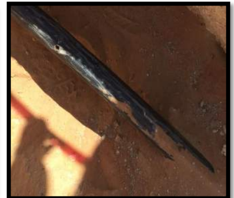
Figure 2.3.6 fault of the cable
