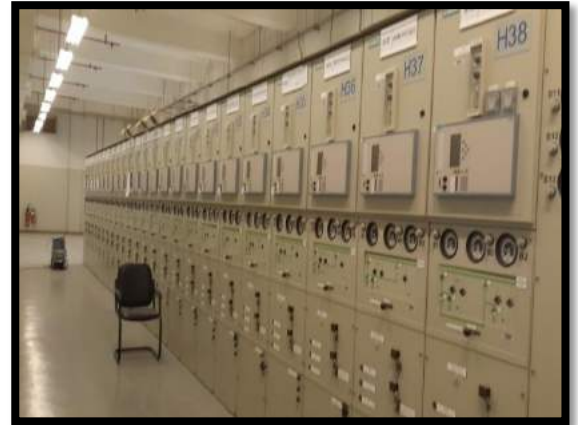
Fig 2.1.3 Grid station, 33KVswitch gear
